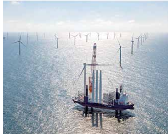
Figure 18. For the 150 monopiles for the Gemini offshore wind farm, Sif relied on the quality of Dillinger's TM plates.
