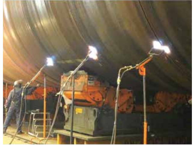
Figure 8. Up to four circumferential welds are made simultaneously by four welding heads, which are controlled by a single system operator.
