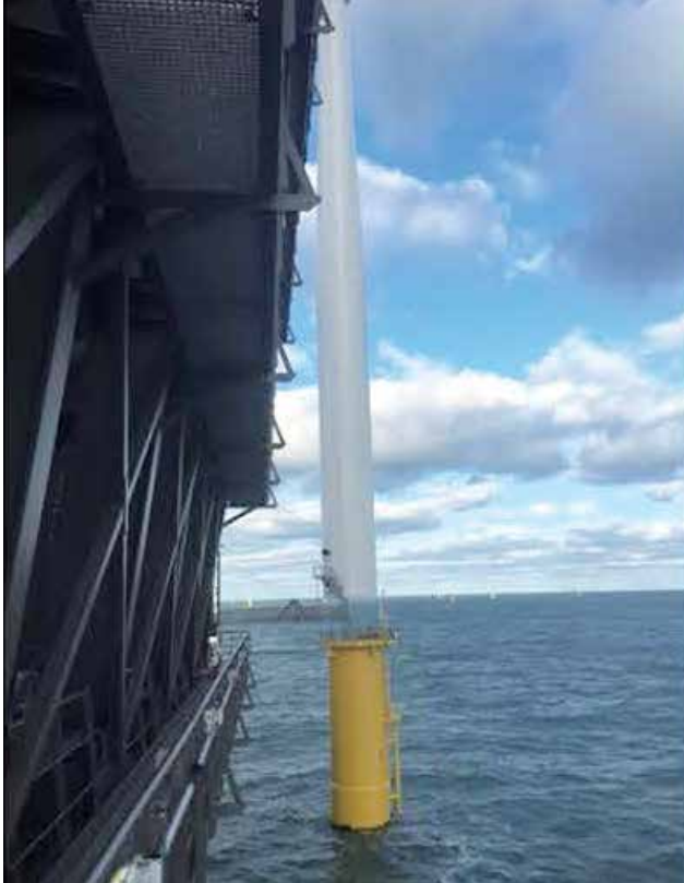
Figure 17. Wind turbines with a rotor diameter of 130 meters were installed on transition pieces made of Dillinger steel.
