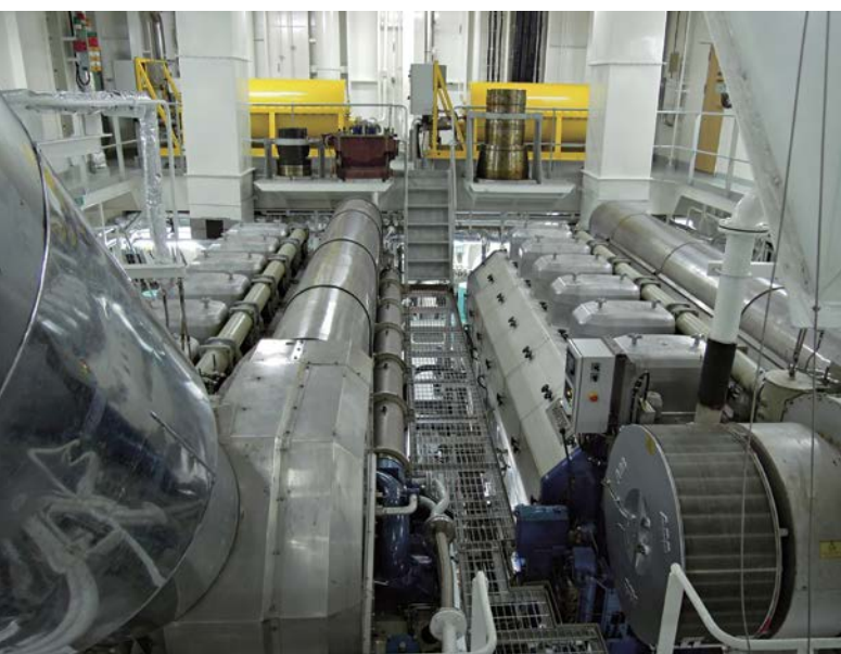
The various systems are fully integrated to achieve maximum efficiencies. Complete propulsion plant delivered by Wärtsilä including CPP, 2 x 6L50DF, twin-in single out gearbox, 2 x 6L20DF auxiliary gensets.
