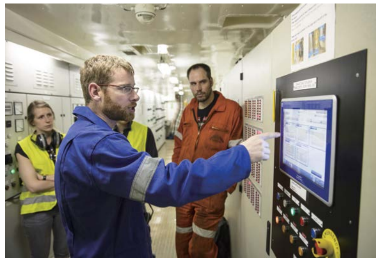
Roland Hooegeveen. Technical Support Engineer at Spliethoff controls the Alfa Laval PureSOx.
