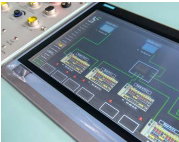
Visualization of the heeling system which allow ships to be optimally trimmed in the water.
