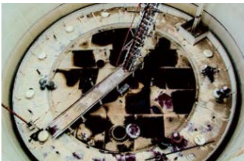
Manual inspections and personnel entering the roof are risky and costly operations
