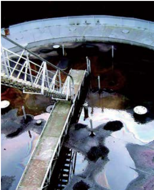
A malfunctioning roof drain is a common problem which could lead to severe consequences
