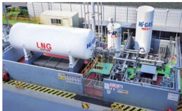
The total LNG carrier demonstration facility built by HHI at its Ulsan headquarters
