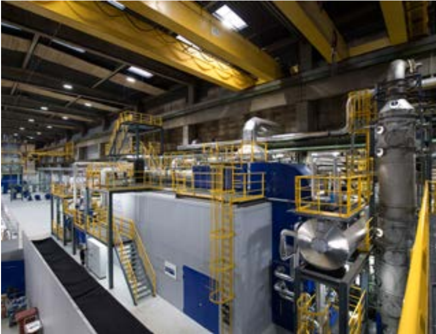
Gas Combustion Unit in the Alfa Laval Test & Training Centre
