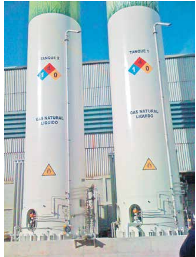
Figure 5. Vertical LNG tanks at a factory in the Dominican Republic. Vertical tanks are used even in areas where hurricanes are common.
