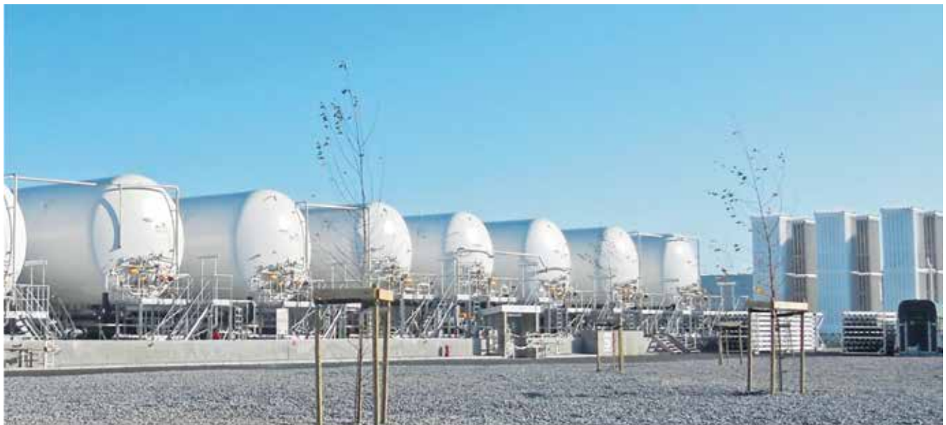
Figure 4. A small scale LNG storage system can consist of a large number of prefabricated tanks. Ambient air evaporators seen in the back on the right side of the image.
