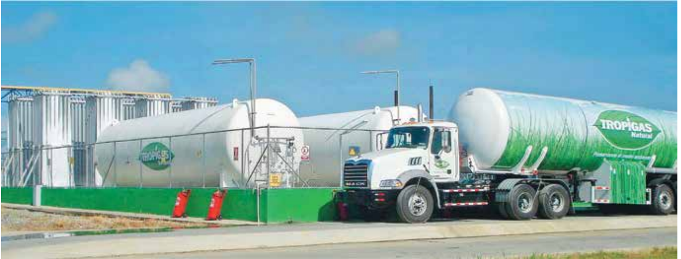
Figure 2. LNG truck unloading at a small two-tank LNG storage facility.
