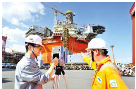
HHI's employees and client's supervisors are using the three-dimensional scanner for the measurement of FPSO under construction.
