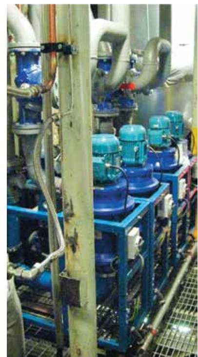
Figure 8. The closed crankcase ventilation units.
