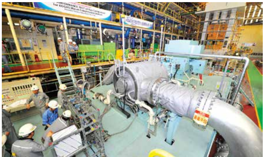
HHI's centrifugal gas compressor of HHI under trial operation
