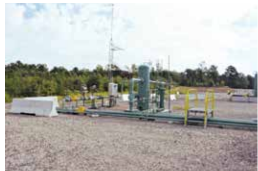
Figure 2. Solar power is often required for remote automation.
