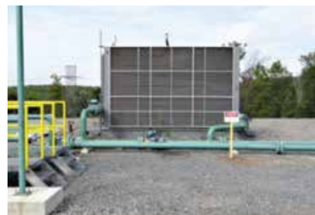
Figure 4. Gas-driven cooler reduces temperature to an acceptable range
