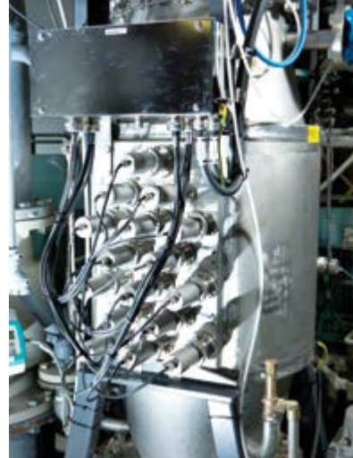
Figure 5. PureBallast 3.0 reactor onboard
