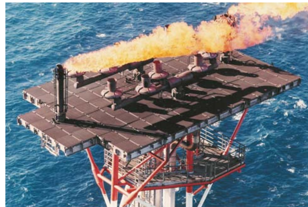
Figure 3. Darflare installation on North Sea platform
