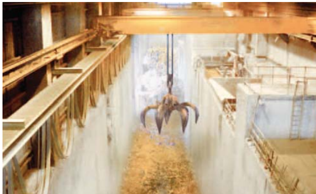
Figure 2. Waste handling crane
