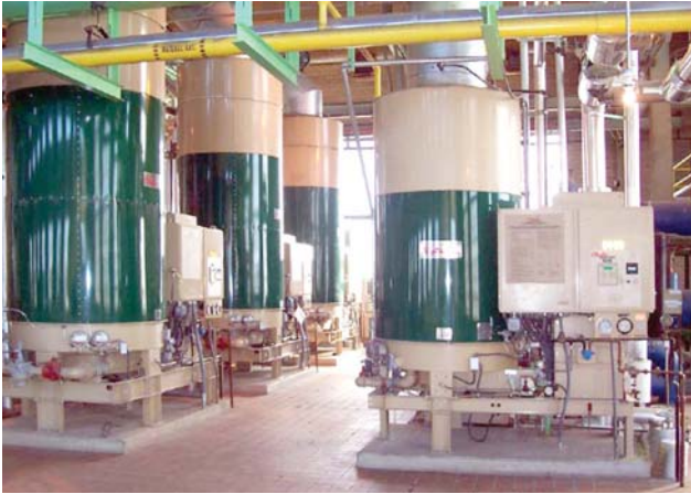
Three 600 BHP and one 300 BHP steam generators in a midwestern utility plant.
