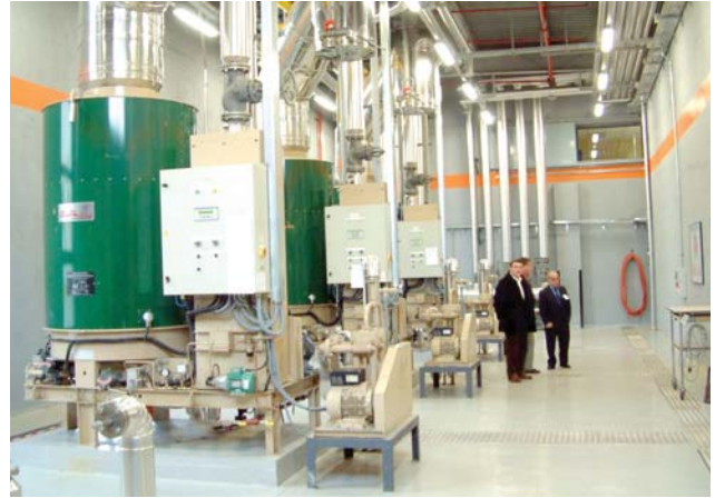
Three 350 BHP steam generators in a Spanish pharmaceutical plant.
