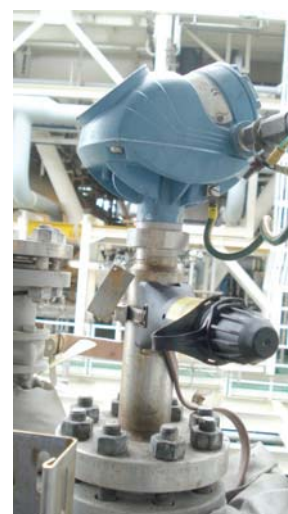
Emerson's Rosemount 5300 Series GWR transmitters have helped BP Exploration increase safety, reduce shutdowns and increase production.
