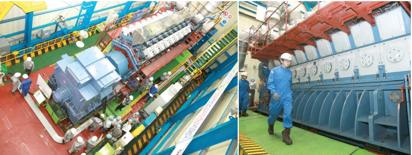
Trial operation of 'HiMSEN' gas engine
