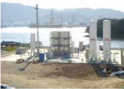
Fuel gas compressor package test facility
