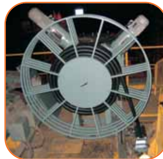
☞ Cable reel installed in Hyundai Hysco
