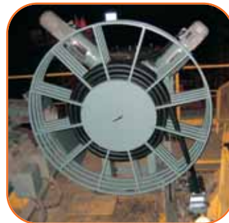
☞ Cable reel installed in Hyundai Hysco
