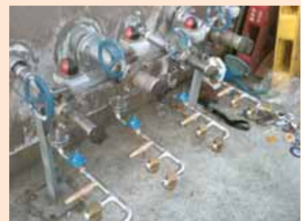
Anti-Freezer installed at port
