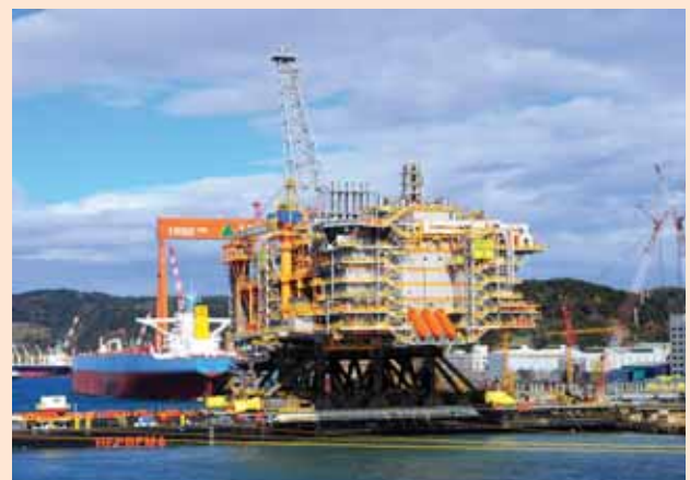
23,000-ton NR2 ultra large offshore platform built by HHI for Australia-based Woodside Energy
