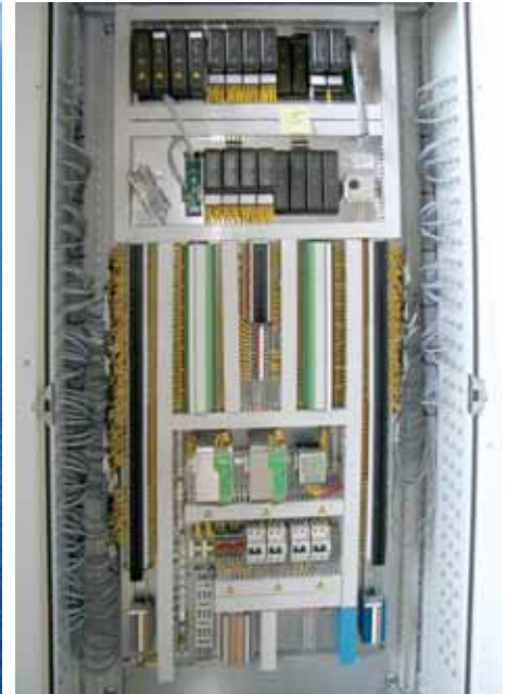
Fig. 2 The control package was integrated in the HPU package and under went factory acceptance testing before being shipped.
