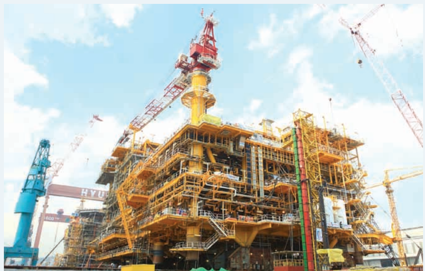
Gas pressurization/refining offshore platform built by HHI, which will be installed in Bongkot, Thailand
