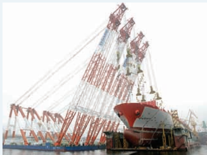
An ultra large block is loaded by connecting 2 units of 3,600-ton cranes in parallel
