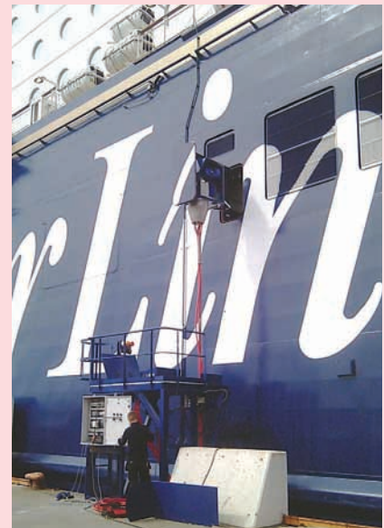
Recently, Nexans announced that it would supply specially-designed power cable to NG 2 for its plug shoreside power system enabling high voltage power link between onshore location and ships through the pushbutton operation.
