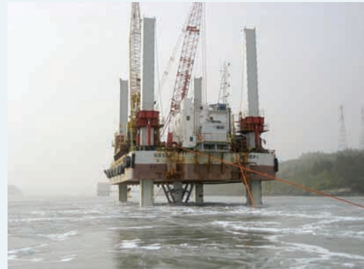
Tidal site for current wind power system installed by HHI in Uldolmok Strait, Jindo
