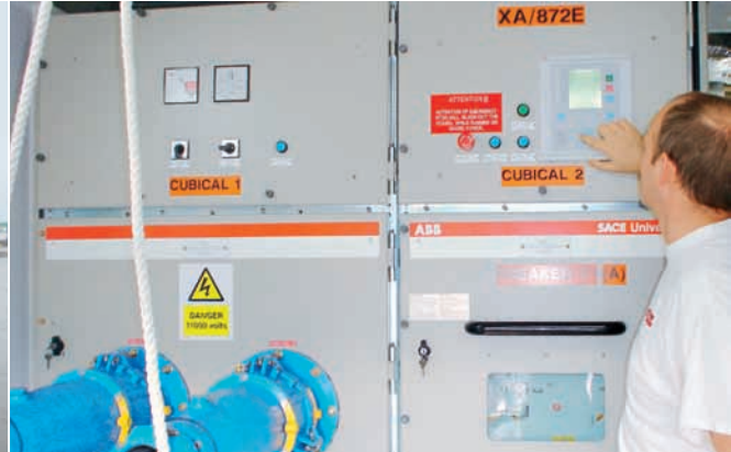
Fig.6 ABB shore connection panel
