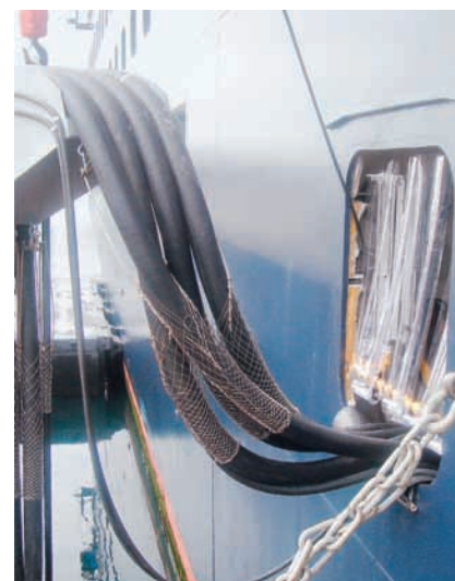
Fig.4 Connection cables on Holland America Line's Vista-class ms Oosterdam vessel
