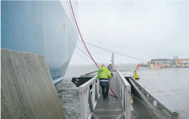
Fig.5 ABB shore-to-ship power connection in Gothenburg, Sweden
