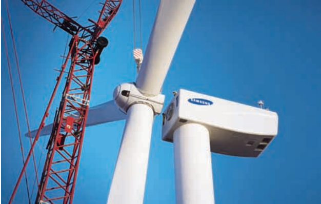
Installation of SHI's first wind turbine installed for the first time in Texas, United States, in 2010
