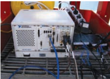
Fig.2 PXI chassis installed at the site
