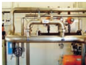
Redox and pH value measurement in a pipe
