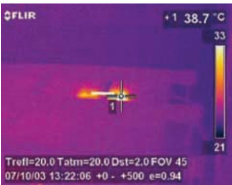
Visual and infrared image of a trip and supply panel
