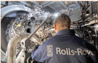
Rolls-Royce powered turbine generator
