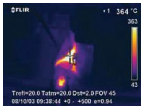
Visual and infrared image of a diesel generator
