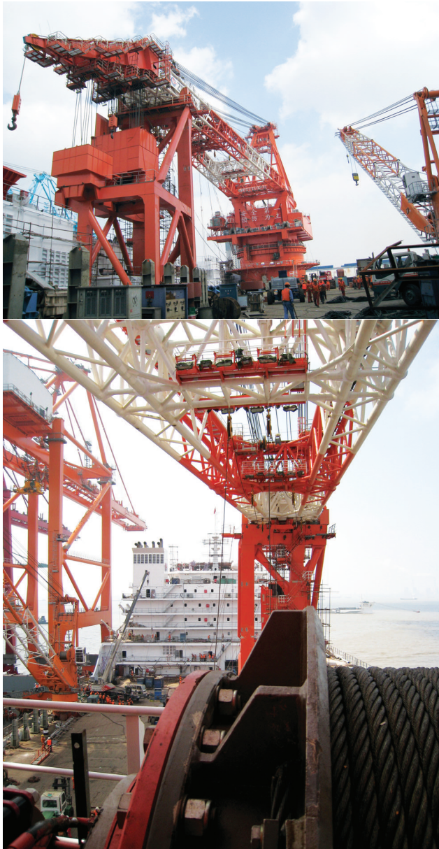
This large derrick pipe-laying barge uses the world's most advanced pipe-laying technology and can lay two pipes simultaneously. The vessel is under construction on Changxing island near Shanghai and will be completed in 2010. Vacon AC drives will also control similar cranes on two other 3,000-tonne derrick pipe-laying barges to be built. (LOA: 170m, Beam: 46m, Breadth: 13.6)
