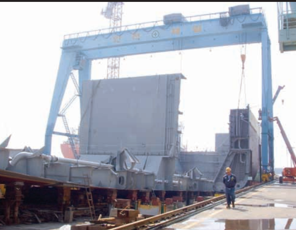
No. H1147~52 8,000cbm ethylene carrier under construction in the No.1 Slipway of the No. 1 Yard (ship owner: Lauritzen Kosan A/S of Denmark)
