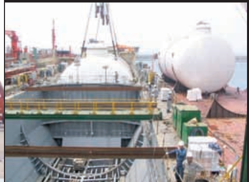
No. H1147 to 52 8,000cbm ethylene carrier TGE gas tank being loaded (ship owner: Lauritzen Kosan A/S of Denmark)
