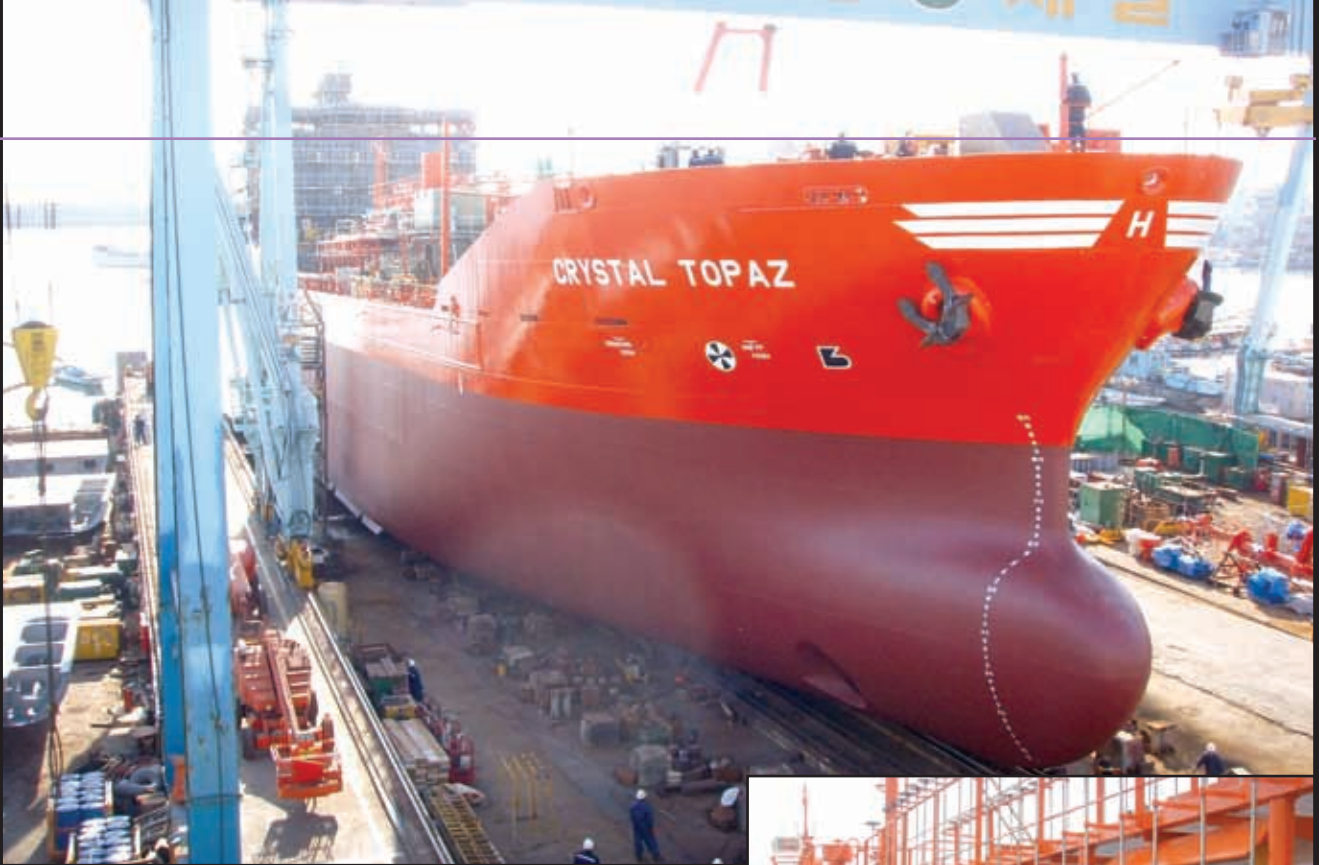
Launching of No. H1139~40 11,300DWT stainless steel chemical tanker under construction in the No.2 Slipway of the No. 1 Yard (ship owner: Crystal Pool Ltd. of Finland)
