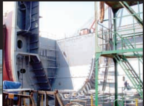
No. H1147~52 8,000cbm Ethylene Carrier under construction (ship owner: Lauritzen Kosan A/S of Denmark)
